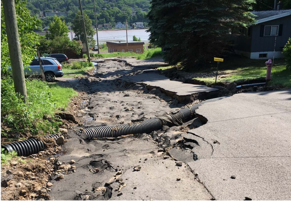
Figure 2-2: Houghton county culvert failure in Ripley, Michigan
