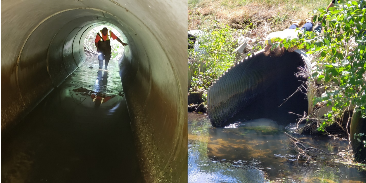
Figure 7-21: The effort needed to inspect and evaluate culverts varied greatly based on conditions
