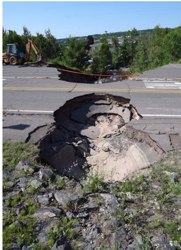
Figure 2-1: Culvert failure in Houghton, Michigan leading to roadway damage
