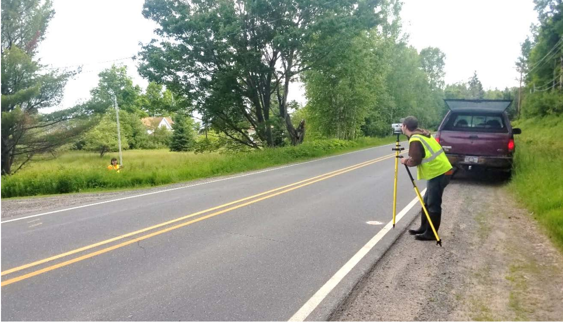
Figure 7-5: Baraga CRC using the auto-level and rod to measure depth of cover
