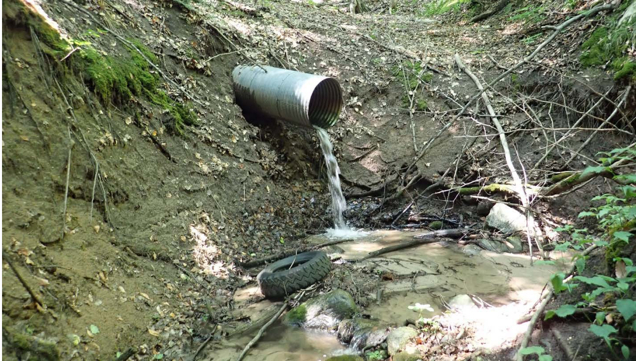
Figure 8-1: Perched culvert which presents a significant barrier to aquatic organism passage. Photo credit Bradley Link, Link Engineering Services, LLC.
