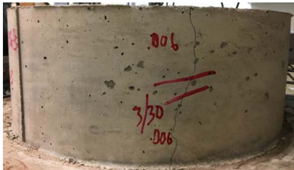
Cracked concrete ring
