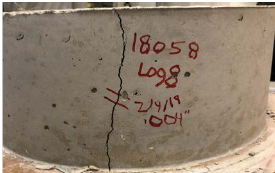
Cracked concrete ring
